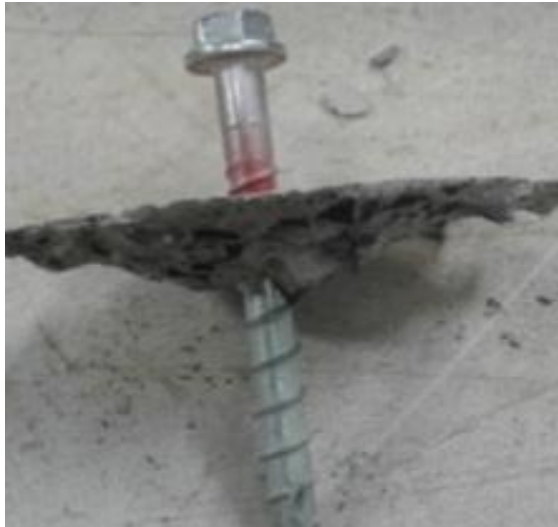
Concrete cone failure
